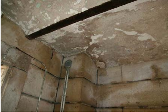
Breezeway below decks, showing impacts of water infiltration. Metal structure and masonry arches will be preserved.
