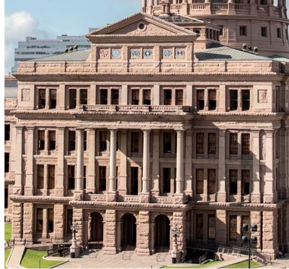
North Portico showing two elevated decks also having tile and waterproofing replaced to protect key historic metal structural elements within.
