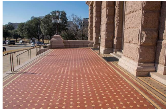
East Deck Today - 1993 era reproduction tile will be replaced, and new waterproofing installed below.
