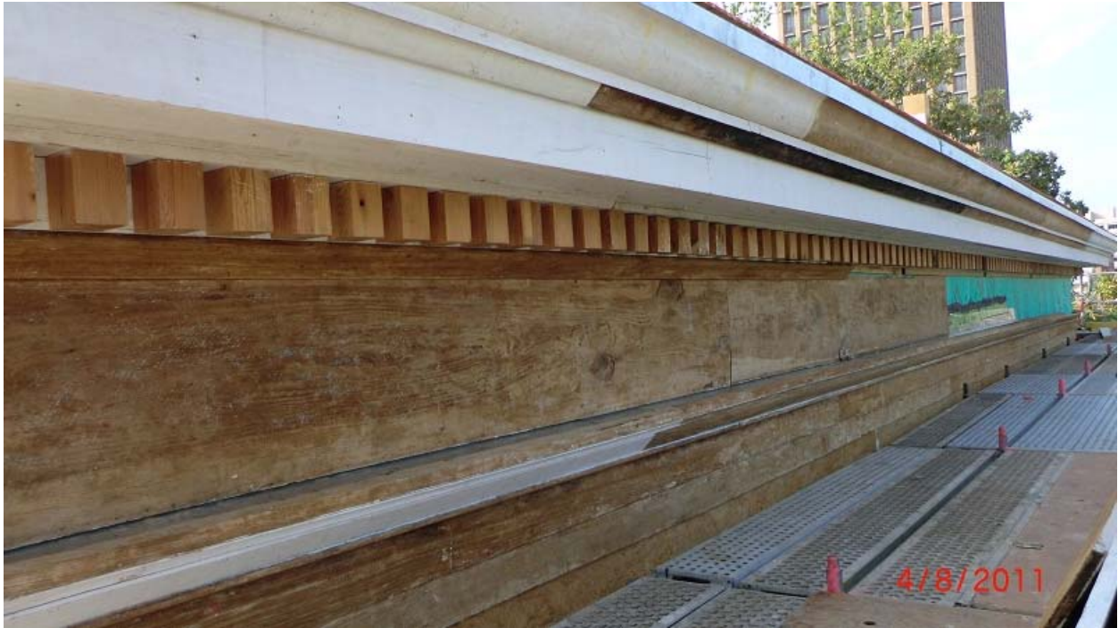
Salvaged wood being installed on the east entablature, along with wood milled from re-claimed beams, for pieces lost in the fire.
