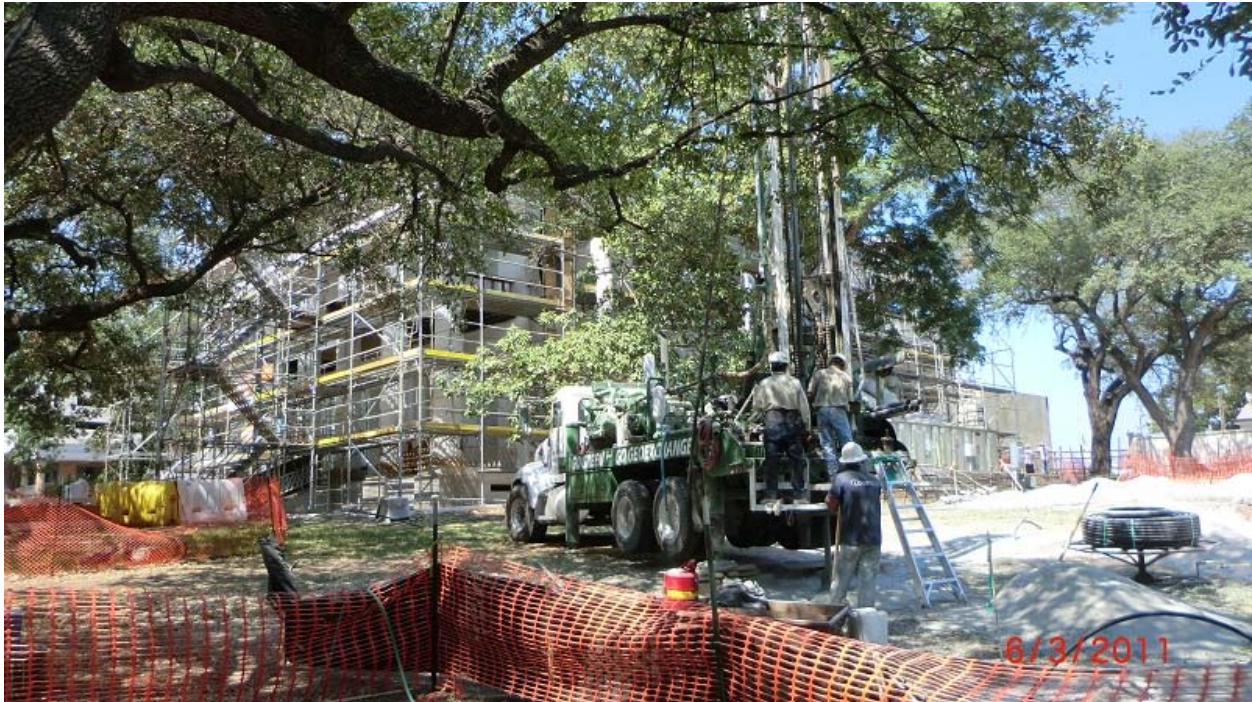
One of 45 wells being drilled on the Mansion grounds, to provide a heat sink and heat source for the home's new HVAC system
