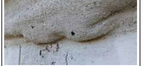
Improper paint application retaining water
