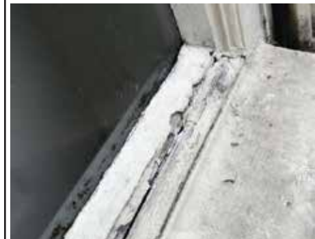
Window glazing and sealant failure
