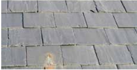
Lifted slates and under or over nailing
