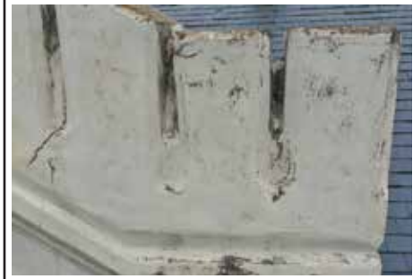
Cracking, loss, and biological growth.
