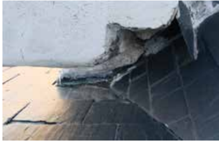
Broken slates and poor slate quality
