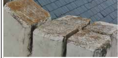
Systemic failure of stucco at water table and projecting horizontal courses.
